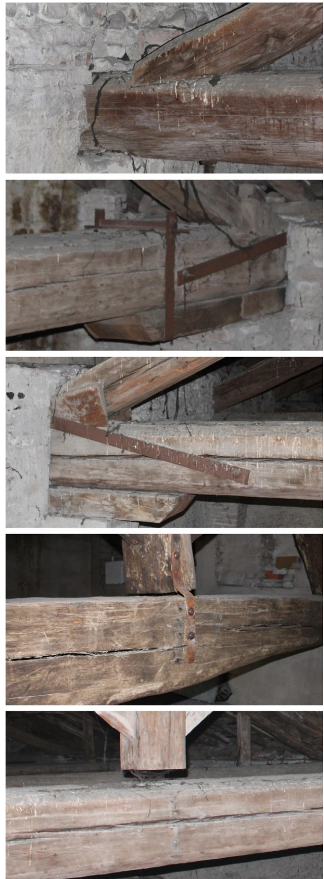
Fig. 2: Examples of different kinds of connections between rafters and tie-beam of trusses and different configurations of king post.
