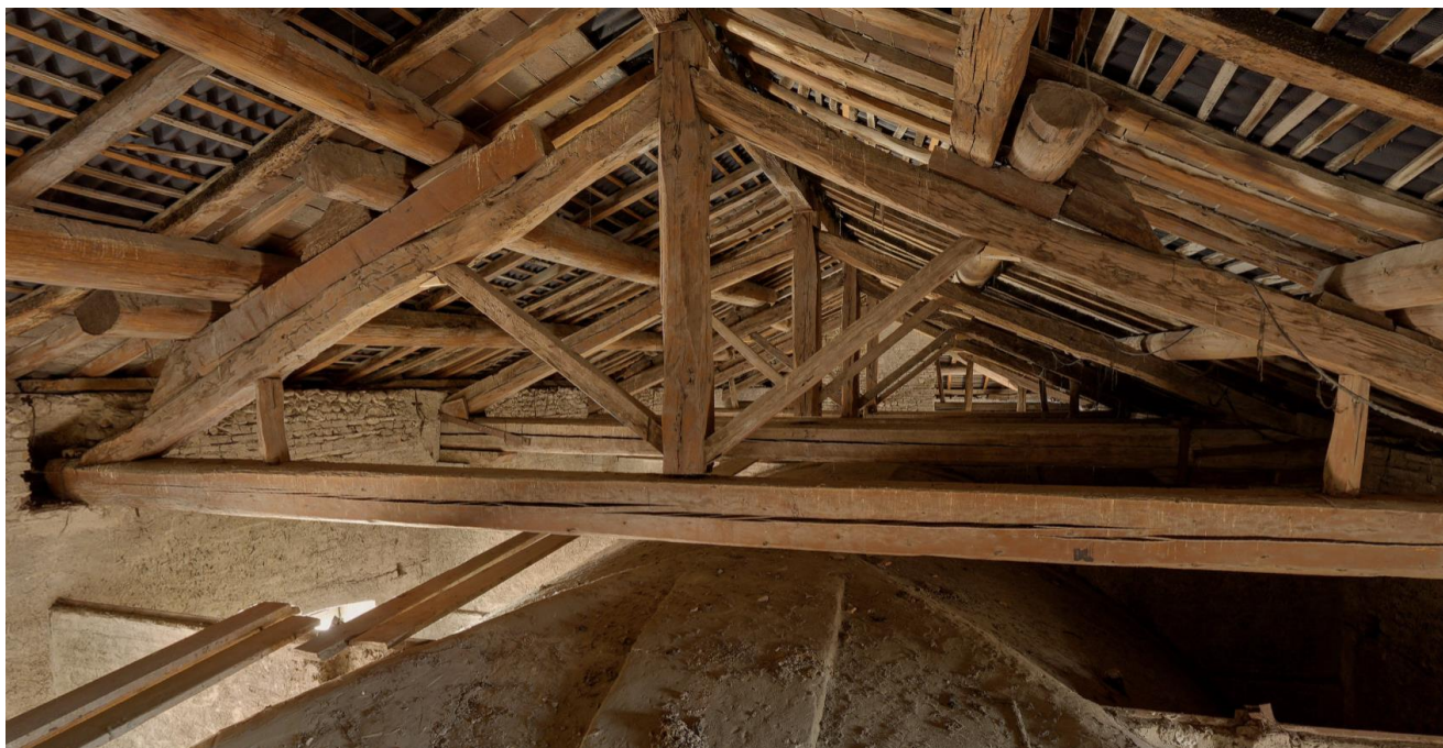
Fig. 6: Photo of the portion of roof of which the H-BIM model was developed.
