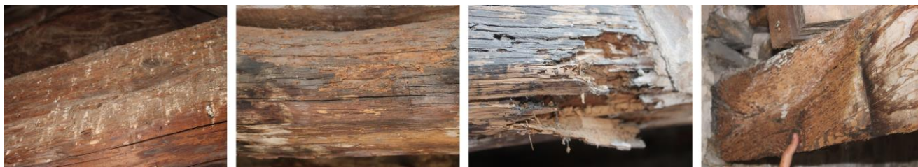
Fig. 4: Different levels of severity of decay. From left to right: level 1-2, level 3, level 4-5, decay limited to beam head.
