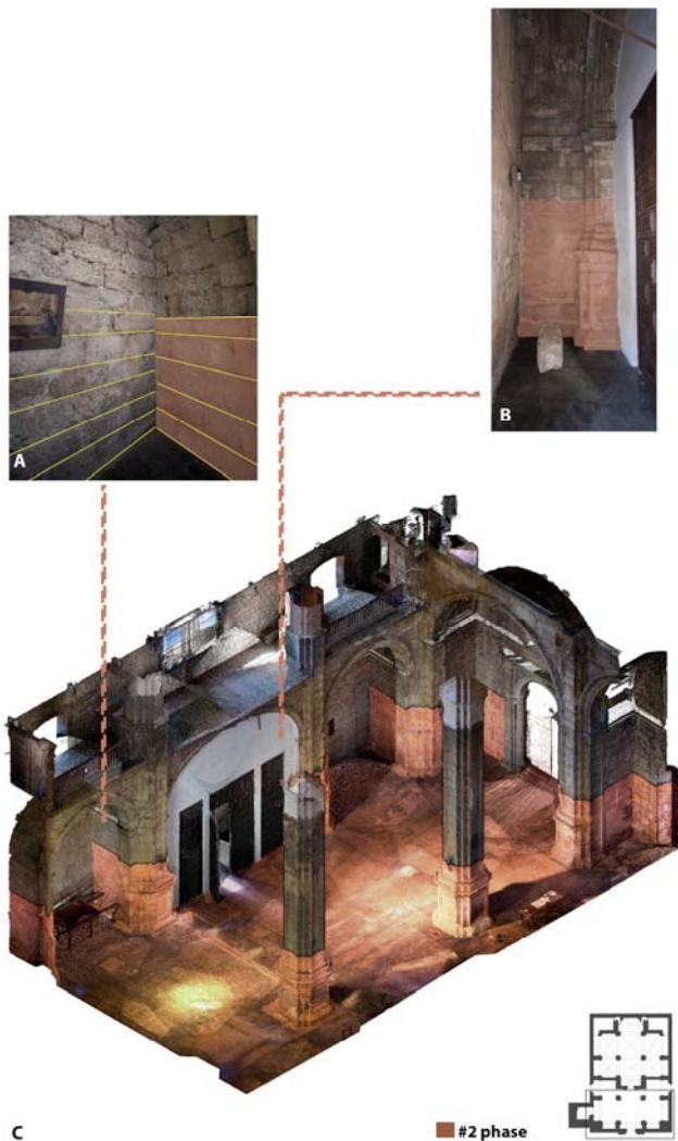
Fig. 10: Foot of the church: (a) lack of bonding between the buttresses and the facade wall; (b) distorted order; (c) perspective view highlighting the 16th-century construction. Author's own.
